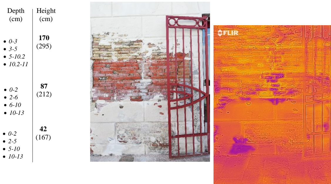
Figure 40 Ex Slaughterhouse San Giobbe masonry in visible and infrared light. The infrared colour scale covers the temperature range between 20-25 °C. Infrared image is shifted with respect to the other one in order to facilitate the comparison by aligning the respective masonry morphological details.
