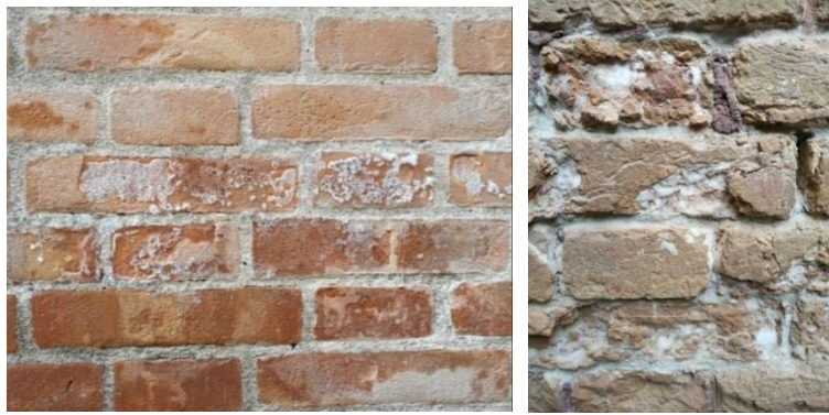
Figure 3 Efflorescence on Venetian masonries. Photos taken on the 25th November 2019 in Sestiere Castello.
